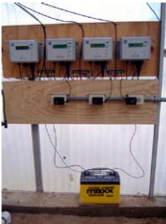
Each raceway was equipped with a YSI 5200 continuous monitor, logging DO and temperature every 5 minutes.
